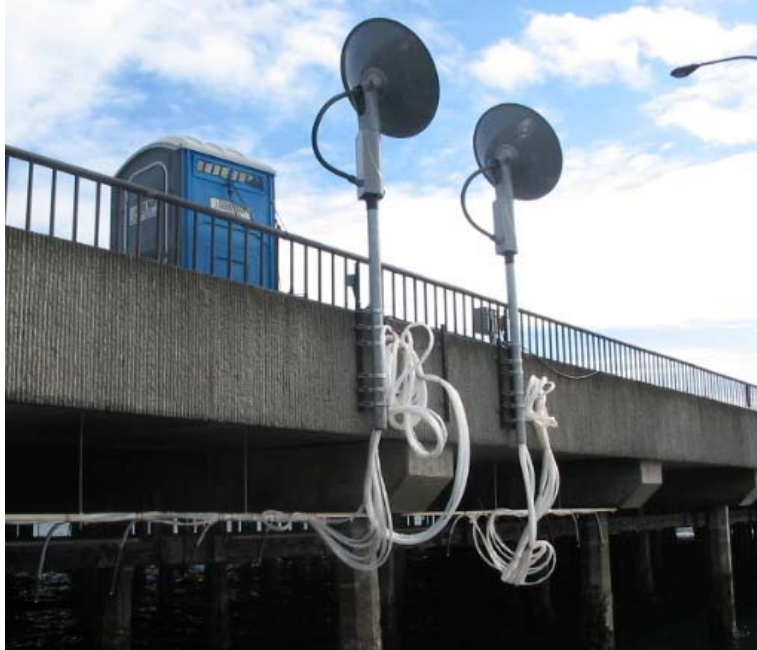
Figure A-1: Image of the fiber optic lighting system. The two dishes above the dock optimize light reception by tracking the sun position, and the cables transmit light underneath the dock.
